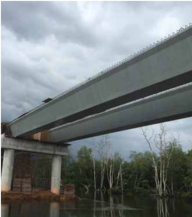
This 10-span bridge connecting Kampung Bahru and Kampung Teluk in Malaysia is shown under construction. Courtesy of J. P. Binard.
