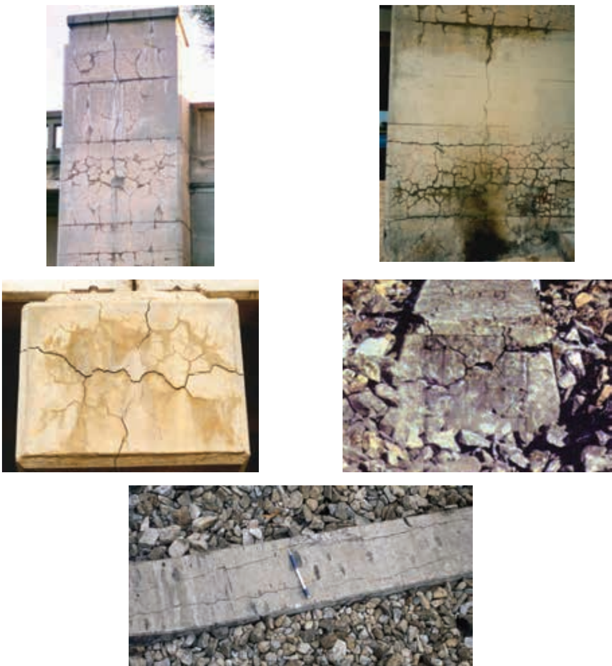
Figure 2: Examples of AAR-induced cracking in bridge pylons (top), crosshead end face (middle left), railway sleeper end view (middle right) and body of sleeper (bottom).
