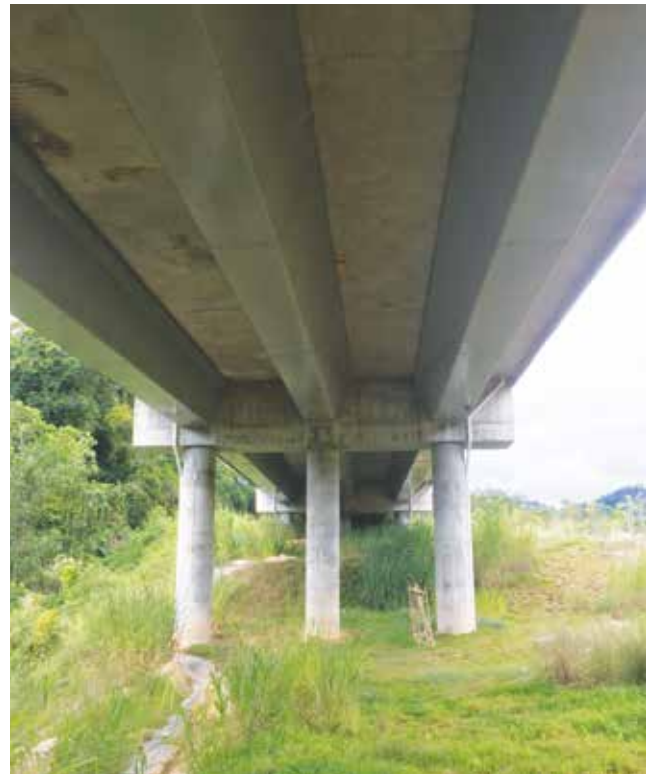
Segmental U beams were used for this five-span bridge along the Koridor Ekologi Central Forest Spine, Gerik, Perak Darul Ridzuan in Malaysia. Courtesy of J. P. Binard.
