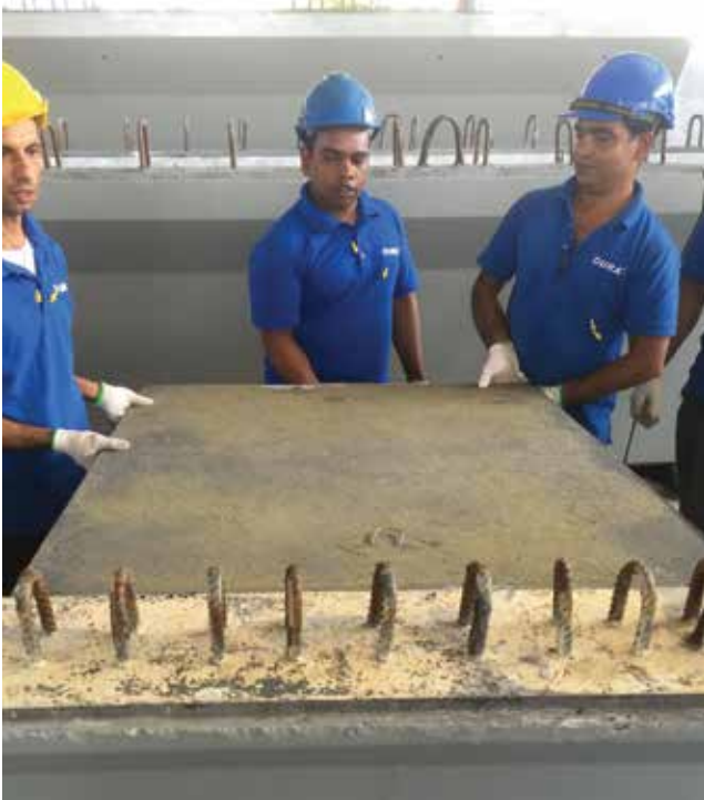
Dura Technology workers use waste ultra-high-performance concrete for a stay-in-place, noncomposite form for cast-in-place concrete deck placement. Courtesy of J. P. Binard.
