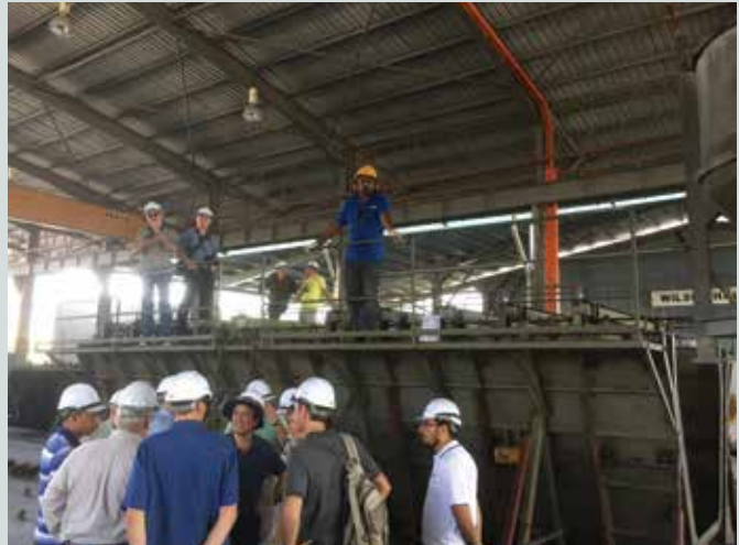
A segmented concrete U beam is prepared for casting with the forms secured and reinforcement present to accommodate horizontal shear requirements for a conventional cast-in-place concrete deck at the at the Dura Technology facility in Ipoh, Malaysia. Courtesy of J. P. Binard.
